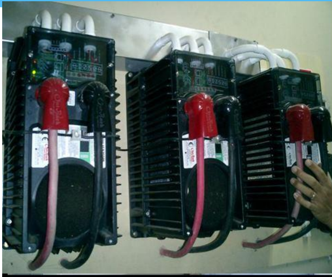
Caribbean's first 3 phase PV System at Green Produce Farms
